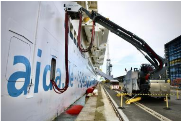
ecological and energy transition, cruise, maritime AIDAnova: first shore power connection in Le Havre for this next-generation cruise ship
